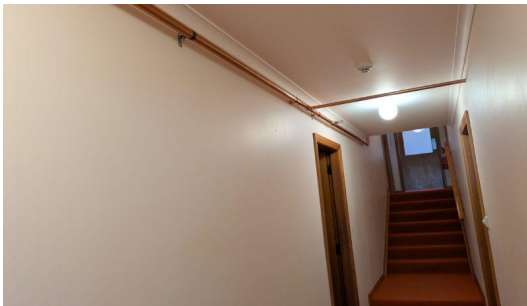
Piping through hallway Level 2.
